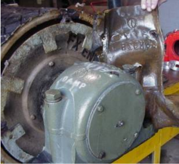
Figure 15: removing CIST material from trial bearing shows impeccable condition of protected substrate
