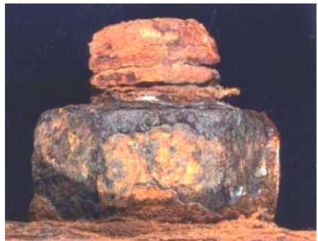
Figure 1: PTFE coated 8 \mu m zinc electroplated low alloy fastener after only 18 months of testing in the splash zone
