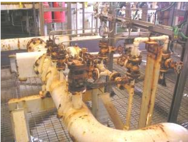
Figure 9: an area of corrosion affected valves
