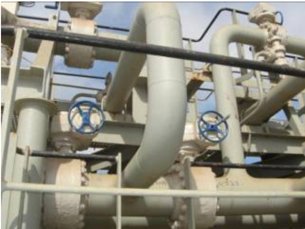
Figure 14: CIST protected deck pipework on LPG carrier
