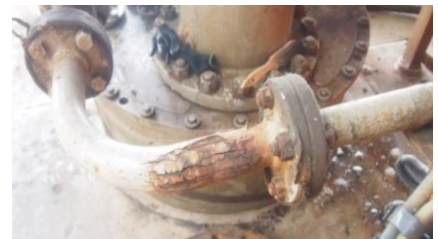
6" Flange & damaged pipe
